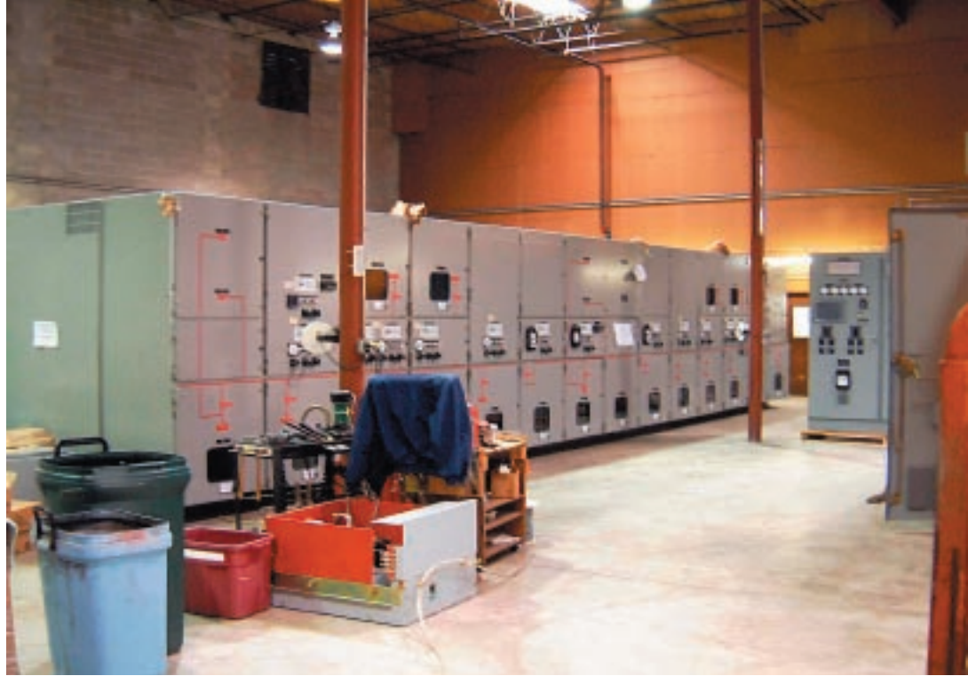
IPS-built Main Switchboards for Bonita Springs Utilities' East Water Reclamation Facility
