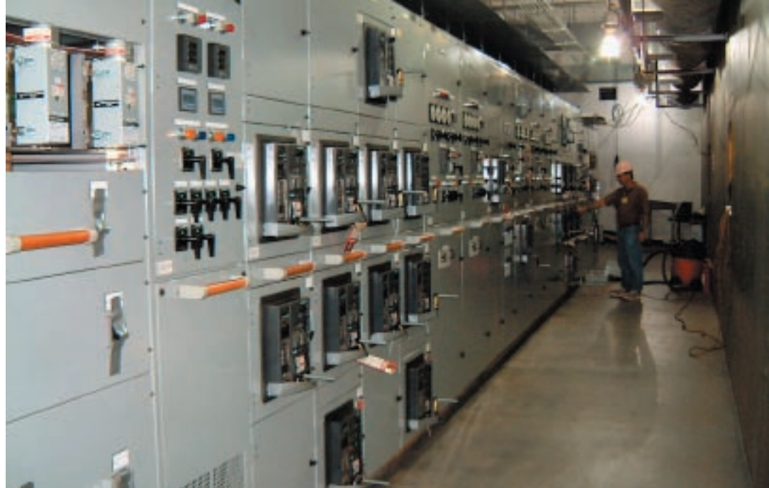
BLUE CHIP 2 main switchboard during initial commissioning by IPS Senior Field Service Technician, Bob Raczak
